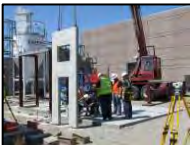
Concrete Tilt-up Lab
