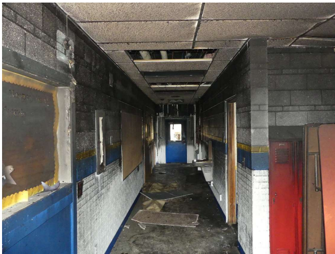
11. Looking north into the north projection from the north-south oriented section of the L-shaped building segment.
