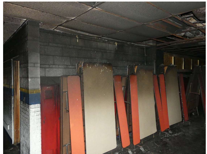
12. Block dividing wall at the north end of the L-shaped building segment.
