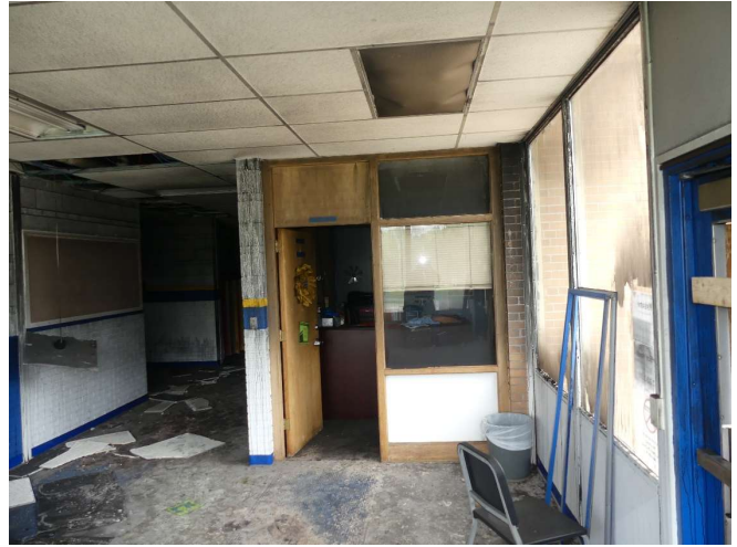
18. Looking north in the foyer at the east end of the L-shaped building.
